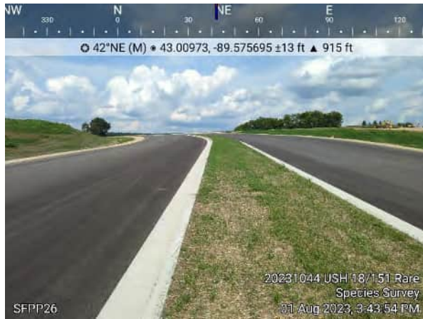
Photo #21 SFPP 26, view northeast of recently constructed extension of Country View Road
